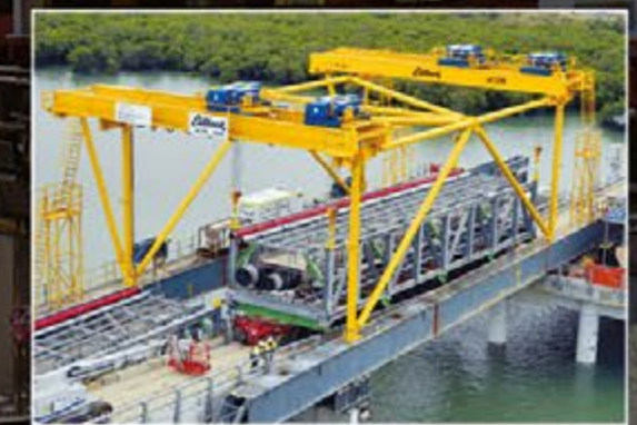
140(50/50/50/50)t Free-standing Gantry Cranes
